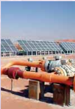
Photovoltaic system at an industrial site
