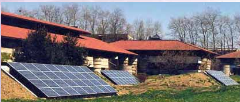
Photovoltaic system at the IUT of Tarbes, France
